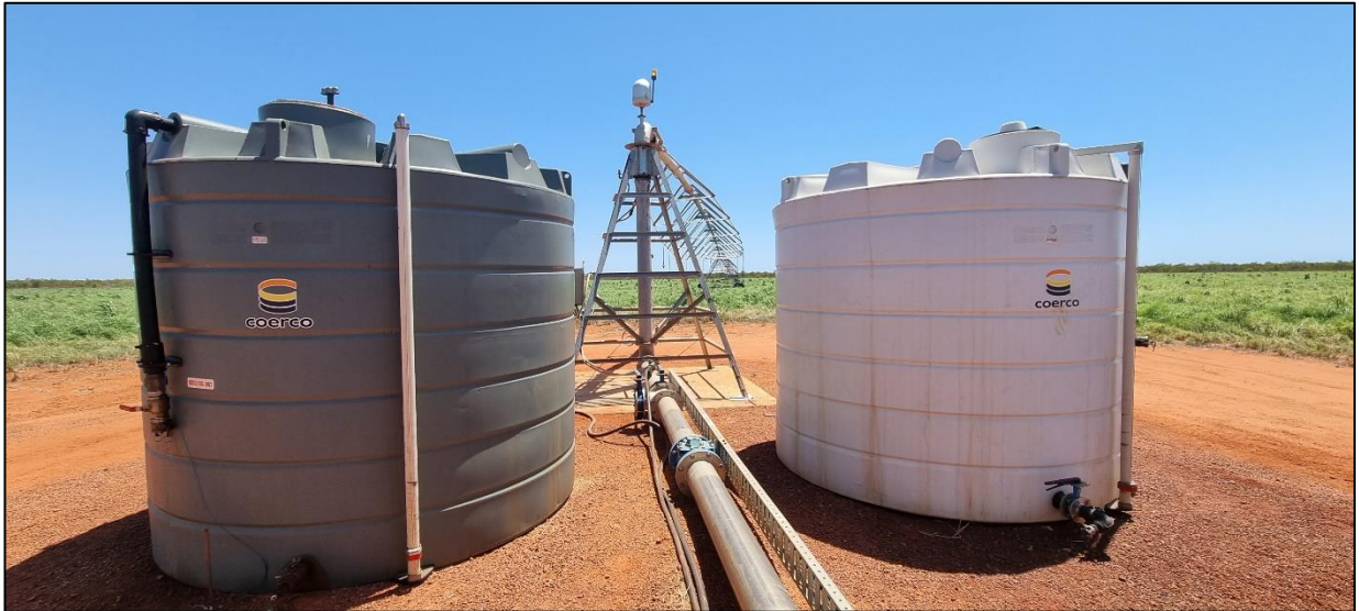
Plate 7 Diesel (left) and fertiliser (right) tanks at Pivot 2
